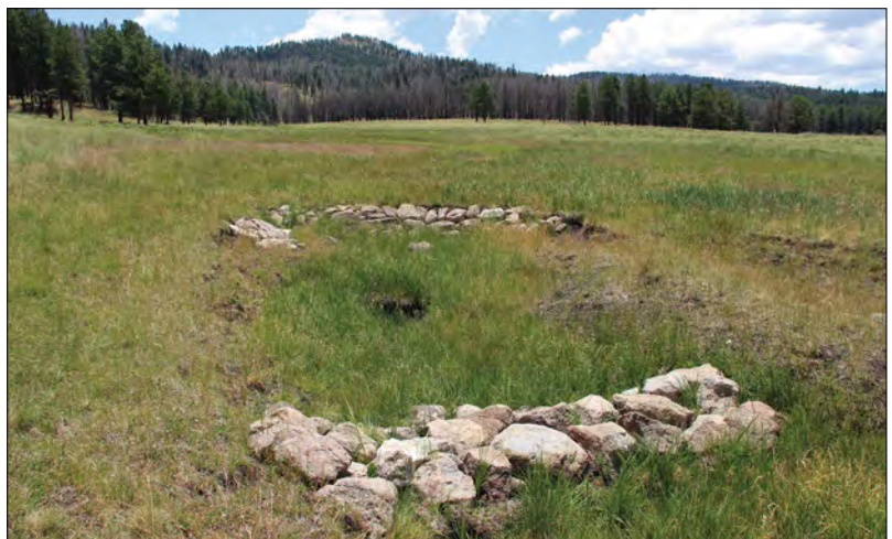
Figure 53. Site 11, July 6, 2017. Paired rock layback and one rock dam as revegetated two years later. (©T.E. Gadzia)
