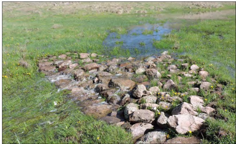
Figure 55. Site 53, May 11, 2017. Rock rundown constructed by volunteers as a stable return site for plug and pond at Site 52. (©W.D. Zeedyk)
